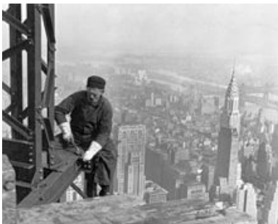
A construction worker atop the Empire State Building as it was being built in 1930. The Chrysler Building is behind him.
