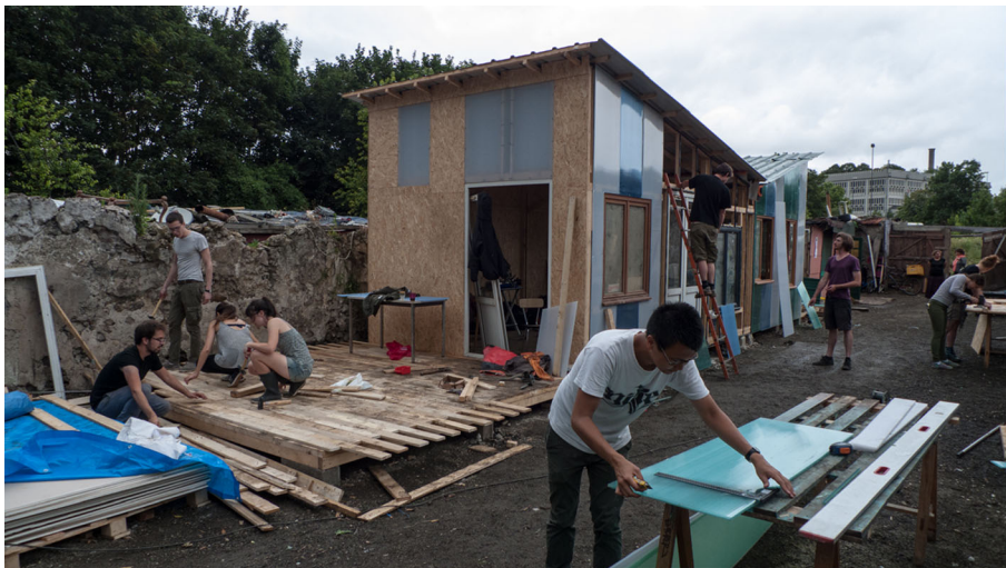
Fig. 1 Students working on the construction of a community building, Montreuil, Paris. The first build, a bathroom, responded to an urgent need that the residents themselves identified. However, a consecutive kitchen project had been offered as a 'gift' to the Roma as they were a 'target group' of the architectural school. This too was problematic as it did not fit with gendered Roma traditions of cleanliness and cooking
