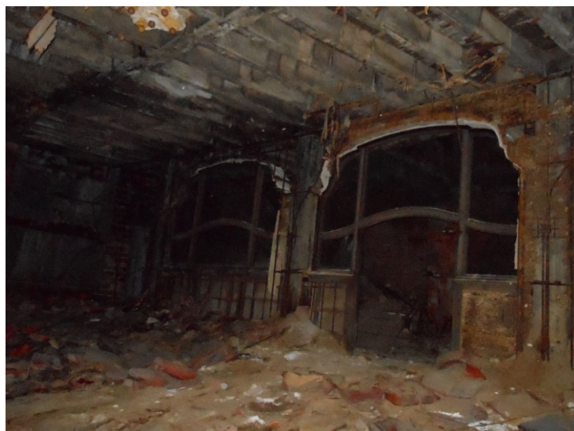
Figure 2. The Palace Theater Lobby, Gary, Indiana (Photo courtesy of Ball State University undergraduate architecture student Shannon Buchanan).
